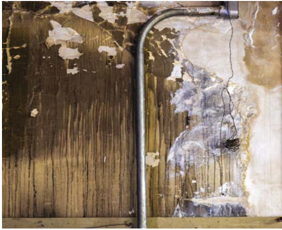
A wall shows the scars of a previous fire.
