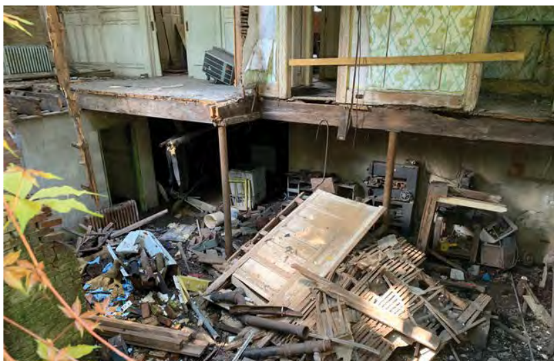
Looking through a hole in the back of the house into the breakfast room/kitchen/dining room. The floors have collapsed so all of that debris is in the basement. A large piece of dining room wainscoting is visible. In the back are the doors to the pantry, the hallway and the pocket doors from the dining room to the living room. (submitted photo)
