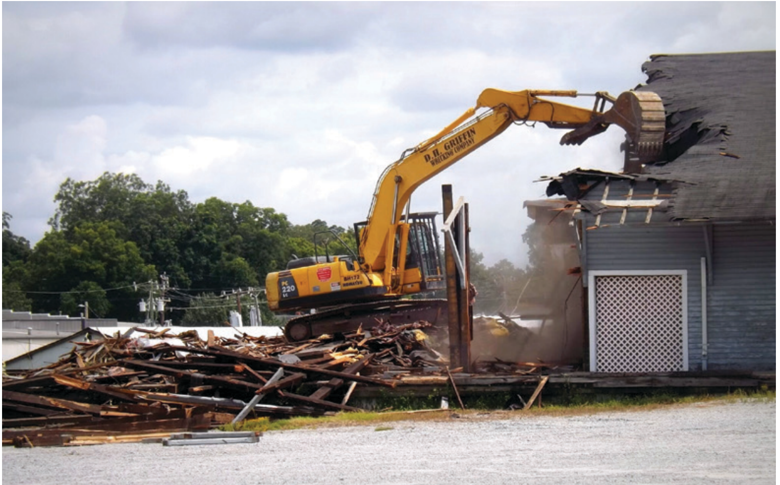
In historic preservation, not everything can be saved. Here, an excavator takes a bite out of Salisbury's old freight depot. Submitted photo.
