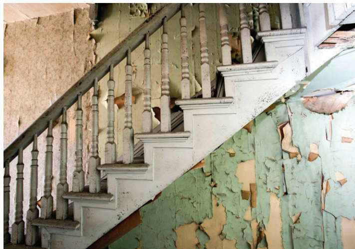
Left: The inside of a wall revealed. Above: Stairs to the next floor. Right: Many of the steam radiators remain.
