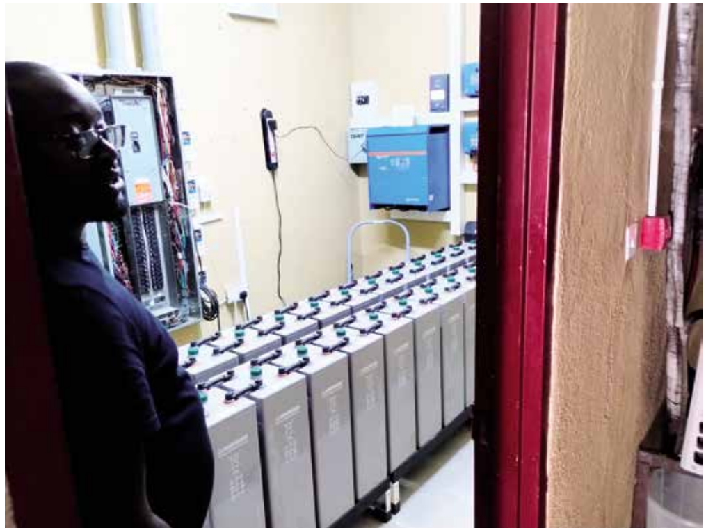
Lawrence Kamba stands next to batteries storing the power from the hospital's solar panels.
